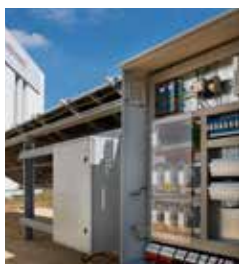
Pv Solar Test Lab
